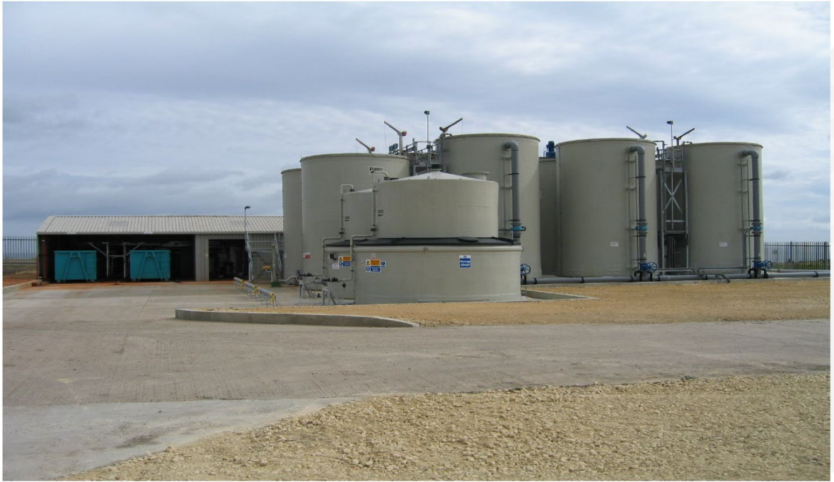
Figure 4-1: Example layout of an HDS treatment plant (Horden Mine Water Treatment Plant, UK)
